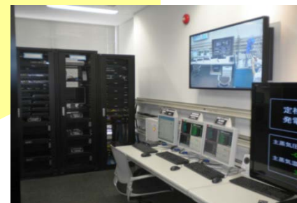
Electric Power Plant
