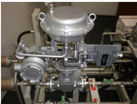
Tank and Valve
