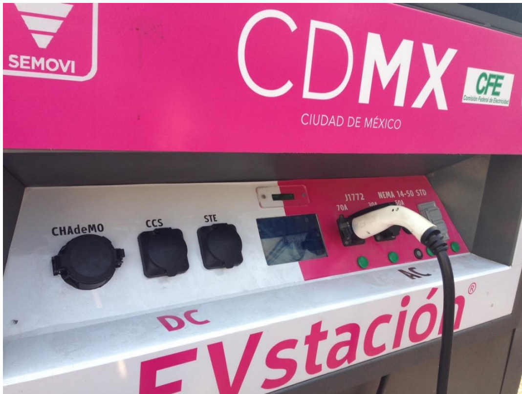
Figure 2.5 - EV charging station in Mexico City with outlets for different charging standards
