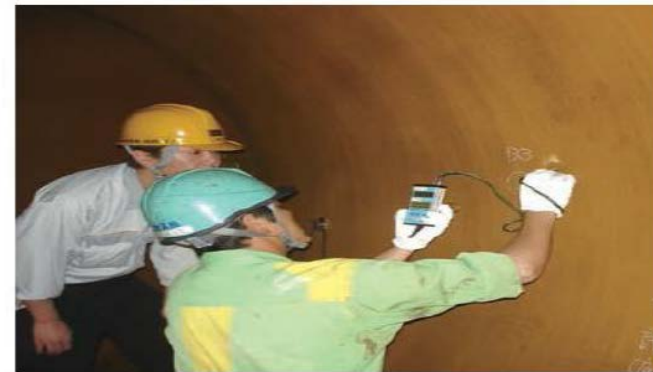
Open-tank wall thickness measurement The thickness of the tank wall is measured from inside the tank for safety verification.
