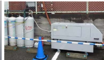
Emergency city gas supply
