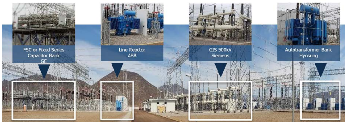
Figure 7 ISA’s ‘Smart’ Transmission System
